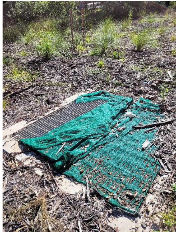
Photo 6 Sediment drain in need of repair in Lot 101 Crest Road
